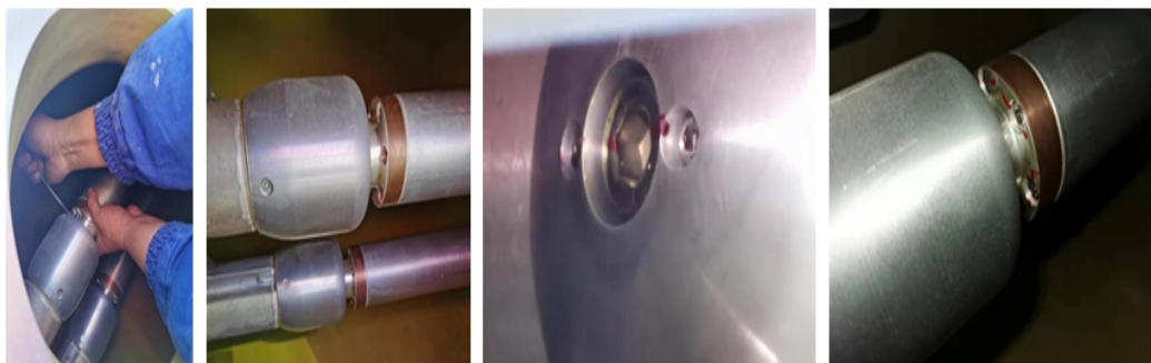
Figure 9 Maintenance maintenance personnel on the site busbar fastening bolt inspection The field test of sectional circuit resistance is qualified.
